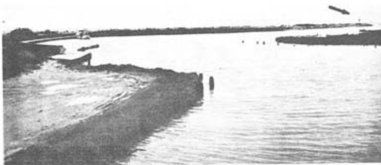
Winnipeg Beach. Note the poor condition of the dock. The sign (A) is a warning. Pole light and daybeacon (B).
